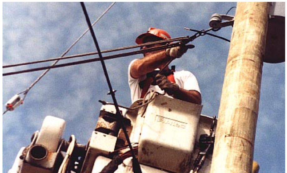
Line workers install, maintain, and repair power lines that carry electricity from generating plants to users. Photo by CGP Staff
