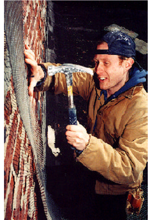
Lathers erect light gauge studs, joists and rafters, and metal framing for lath and plaster and for drywall. Photo by Amy Elliott
